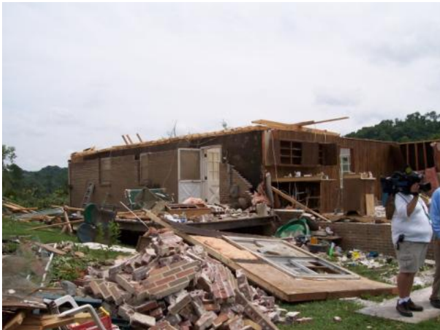
Figure 1. Tornado damage in Giles County. (Photo courtesy of National Weather Service)
